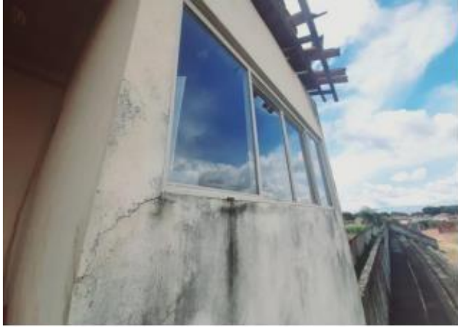
19 – Vista frontal lateral cabine radio
